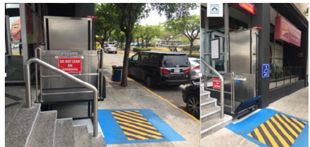
Figure 2: Wheelchair lift installed by Comfortair Engineering Limited at the First Caribbean International Bank Building.
