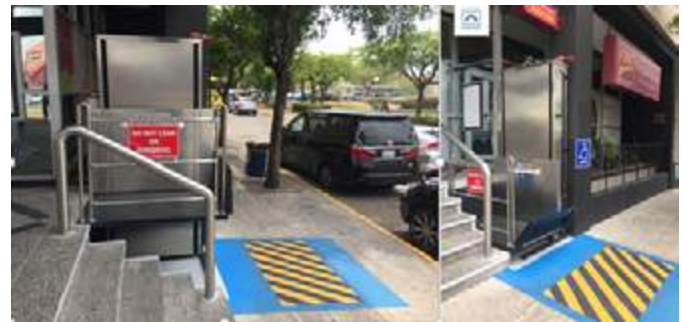
Figure 6: Wheelchair Lift intalled at FCIB building in New Kingston by Comfortair Engineering Ltd.
