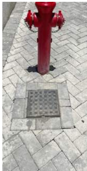
Figure 5b: Fully commissioned fire hydrant.
